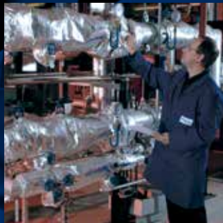
Ready assembled control systems
